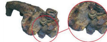
Starke Korrosion / strong corrosion
