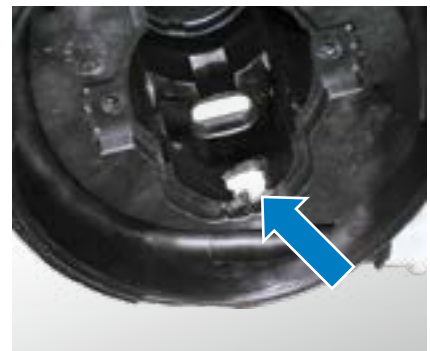
Damage symptoms: Melting traces on the housing (top view into the housing)
